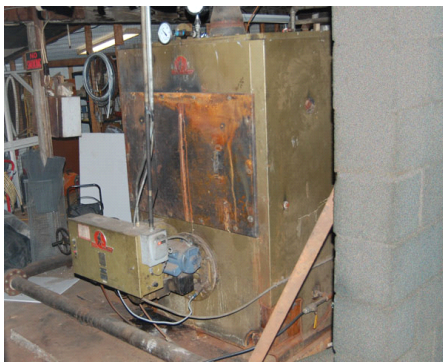
Pictured: Newer boilers are made with noble metals like copper and stainless steel, which don’t rust and corrode. Photos courtesy of BioTherm.
