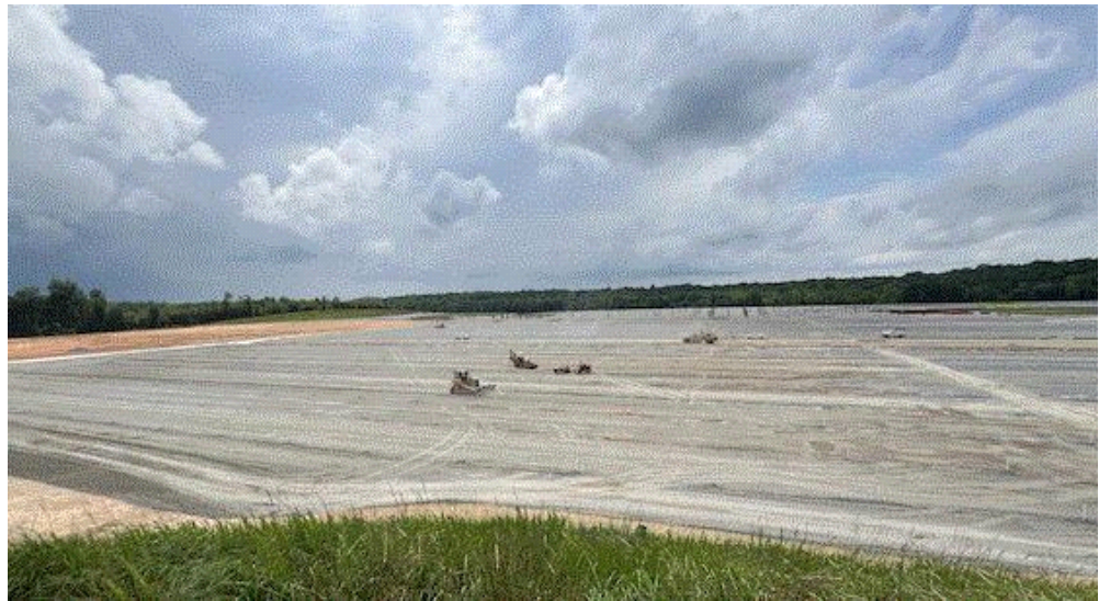
Metrolina was just finishing up an 88-acre outdoor addition that will be filled with fall mums very soon!
